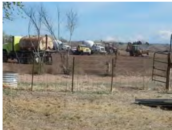
Tractors pulling boat and concrete trucks delivering concrete into boat as ditch is poured.
